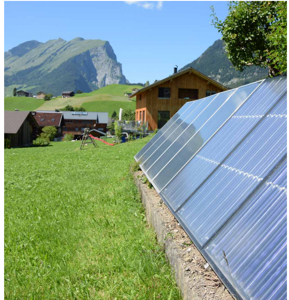
Solar installation © Adobe Stock
